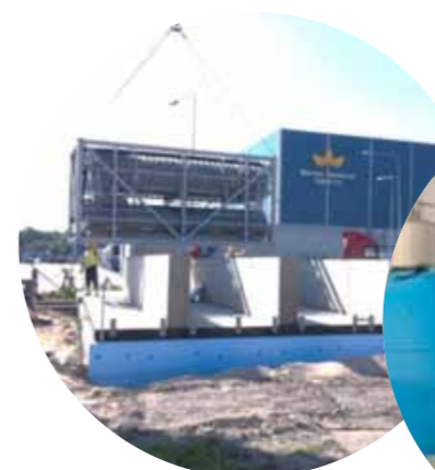
Tobacco factory wastewater treatment in Russia
