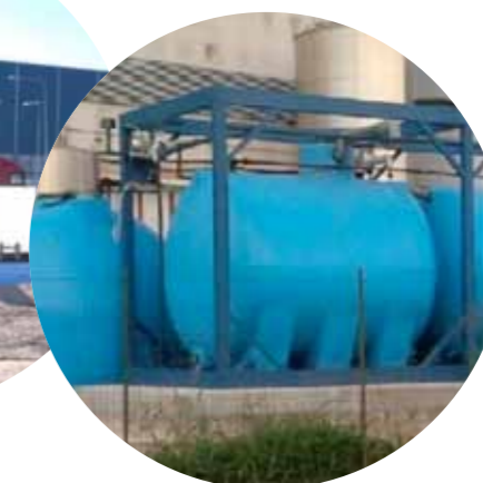
Winery wastewater treatment in Italy
